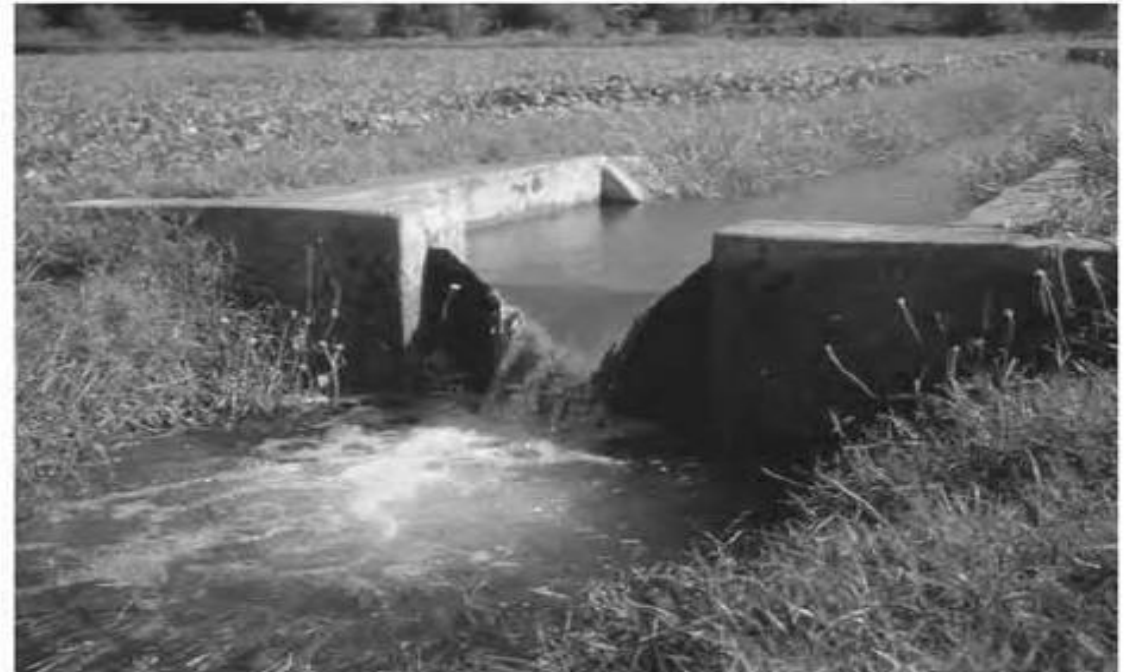
(c) Photograph of a V-shaped weir
